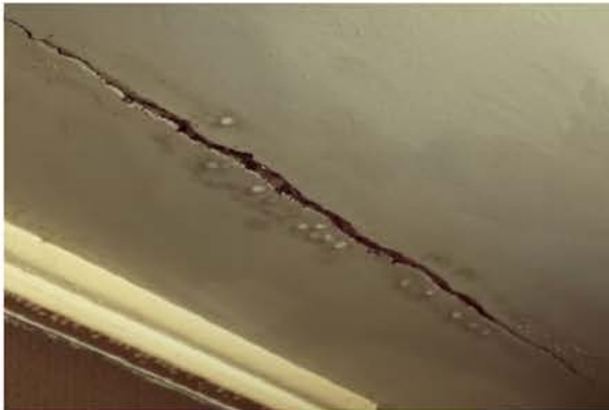
Stock condition surveys are crucial for discovering issues such as damp and mould (picture: ITV)
